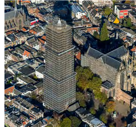
Nico de Bont restores the iconic Dom Church and tower in Utrecht.
