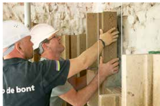
Restoration of the Eusebiuskerk in Arnhem: sustainable value creation by preserving a monument for the future.
